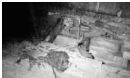
Some of the damage that will be repaired in Baker Lodge
